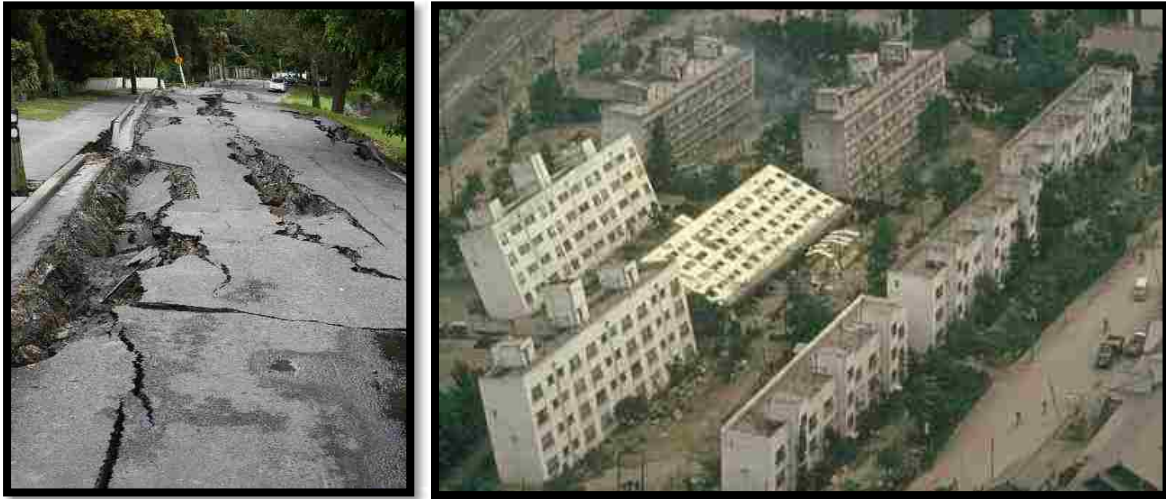
Figure 1: Damage to infrastructure from liquefaction events. (left) River Road, Christchurch New Zealand damaged from lateral spreading in the 2011 earthquake series. (right) A dramatic example of sinking apartment buildings due to the loss of soil shear strength, Nigata, Japan 1964.
